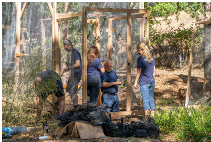
Volunteers from the Nielsen Global Impact Day add more hardware cloth to the structure.
