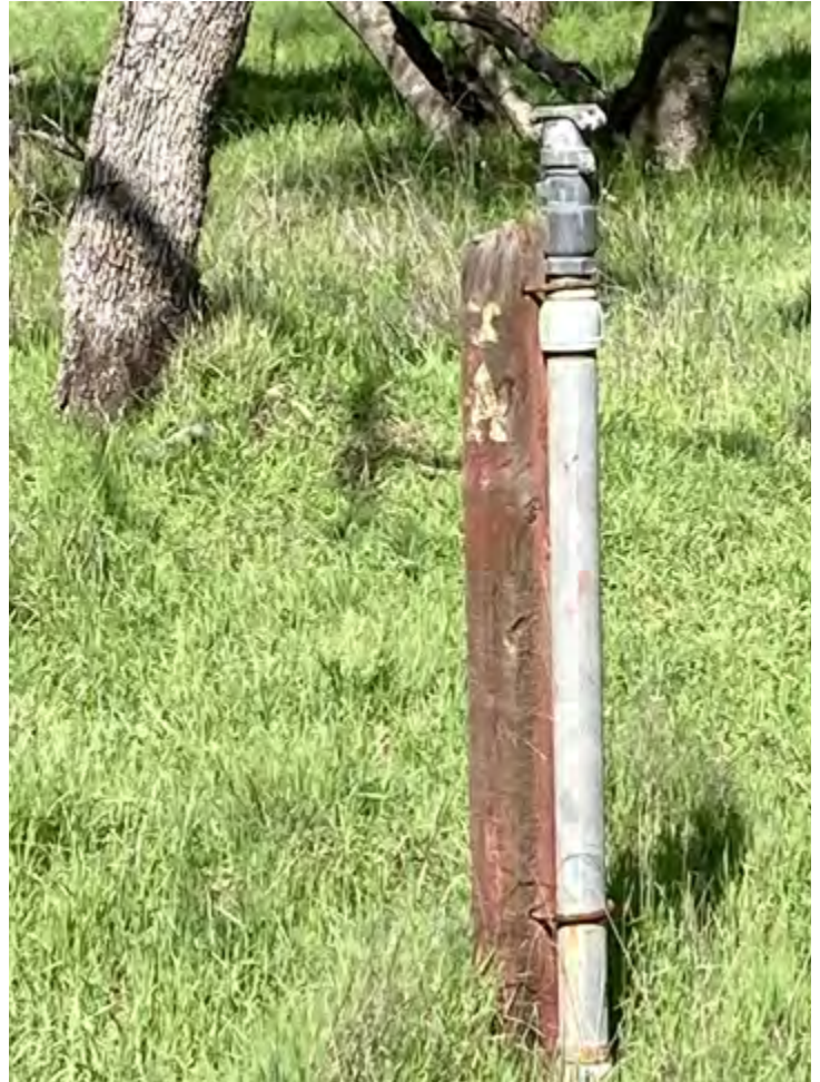
A standpipe that can be accessed to shoot water onto a fire in the NSA. Photo © Melanie Loo.
